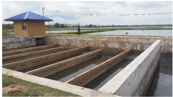
Figure 66: Wastewater treatment plant in Vavuniyakulam (photo credit: IWMI)
