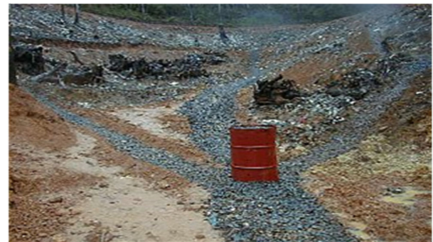
Figure 53: Gas Venting Facility - Moonplains
