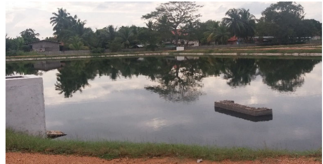
Figure 67: Sewage treatment plant in Thandikulam
