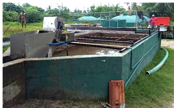
Figure 50: Kurana septage treatment plant
