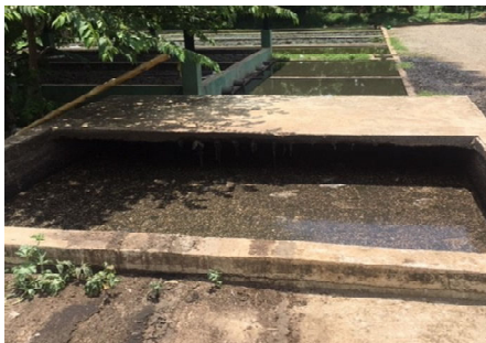
Figure 35: Septage treatment plant at Sundarapola
