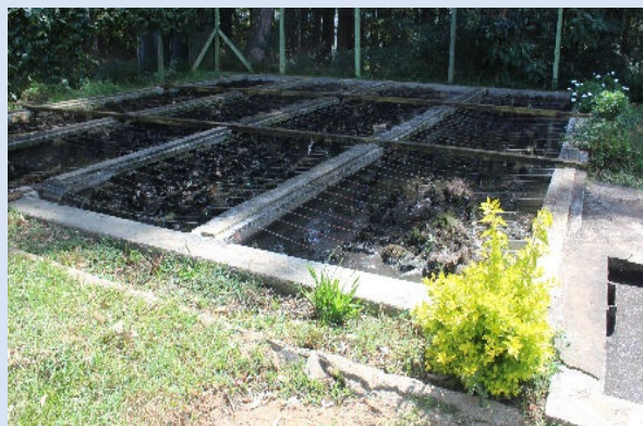
Figure 54: Septage treatment plant in Moonplains
