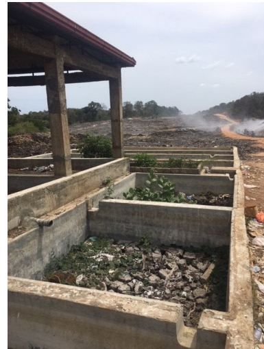
Figure 64: Septage treatment plant in Trincomalee
