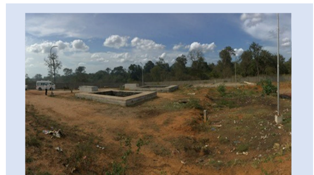
Figure 68: Septage treatment plant in Vavuniya
